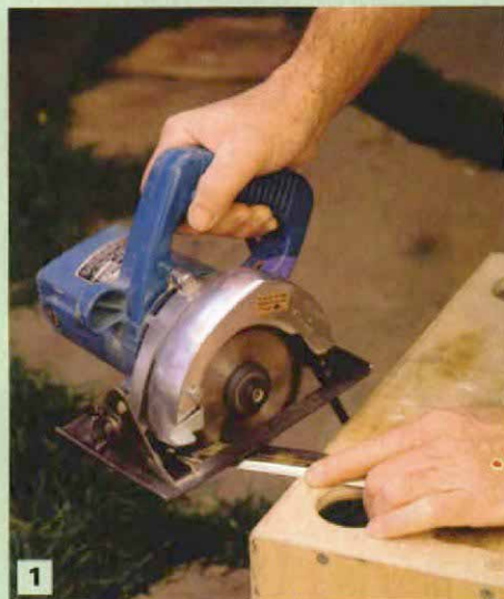
1 Cut rigid jamb with a high-rpm circular saw. A carbide-tipped blade makes short work of rigid-jamb weatherstripping. A hacksaw works, too, but not tin snips. They leave an ugly scar on the metal.
