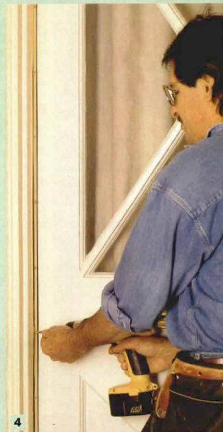
4 Use screws, not nails. Rigid-jamb weatherstripping is adjustable. Drive screws at the top, middle and bottom; then push the strip in to meet the door before tightening.
