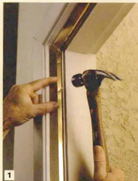
Miter V-bronze in the corners. To avoid overlap, the V-bronze flaps are cut at 45° angles in the corners. The strips on the side jambs are placed ¼ in. away from the stop. Strips of V-bronze are nailed every 3 in.
